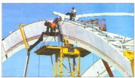
Work continues on the mezzanine roof of the Richmond Olympic oval. Mark Fisher photo
